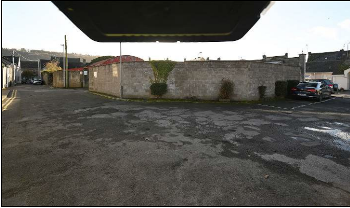
Photograph 3: Northern return to the Depot boundary, looking southeast. A speed ramp table is proposed for here. The concrete block boundary wall will be replaced.
