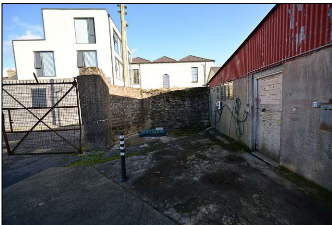
Photograph 7: Exposed stone fabric of eastern boundary wall, south of the entrance, looking east. This fabric will be removed, and requires a photographic record in advance, once the Depot shed is demolished.
