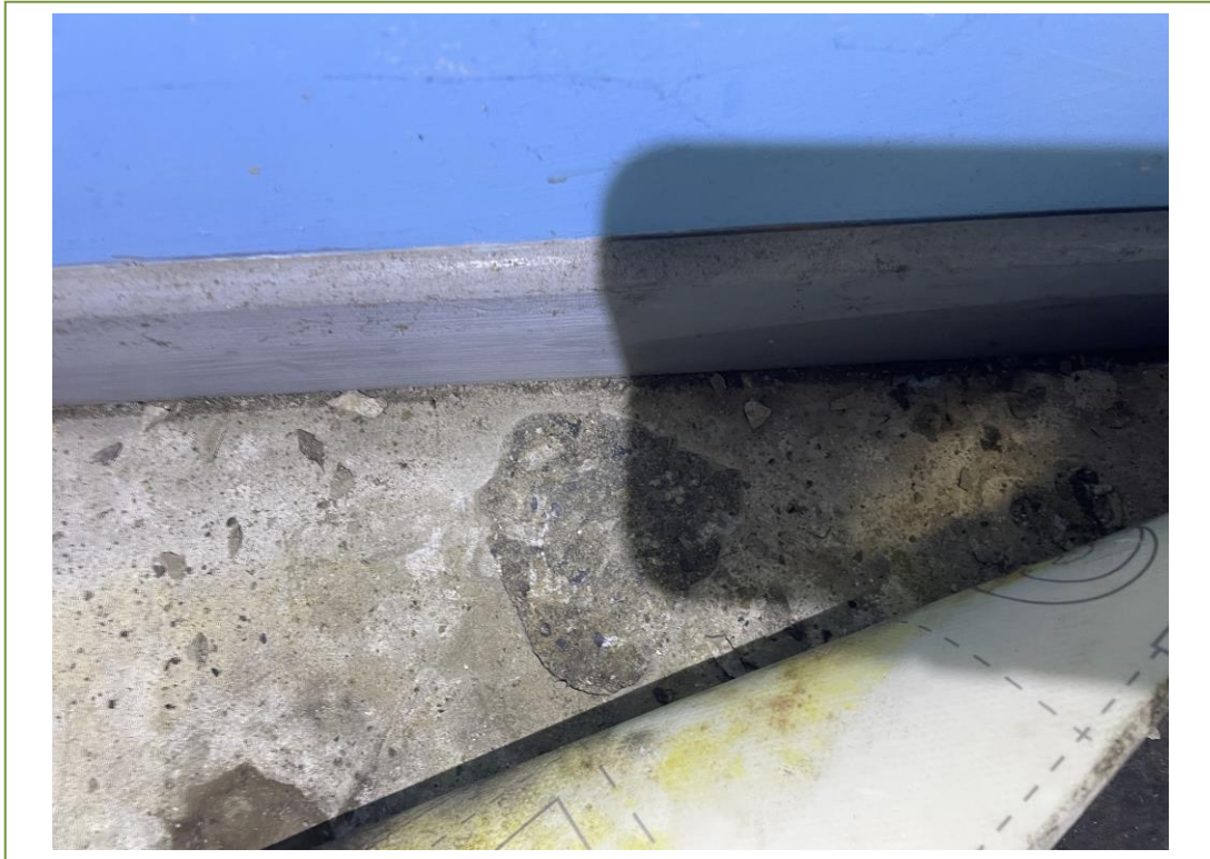
Adhesive under floor covering in the locker room
