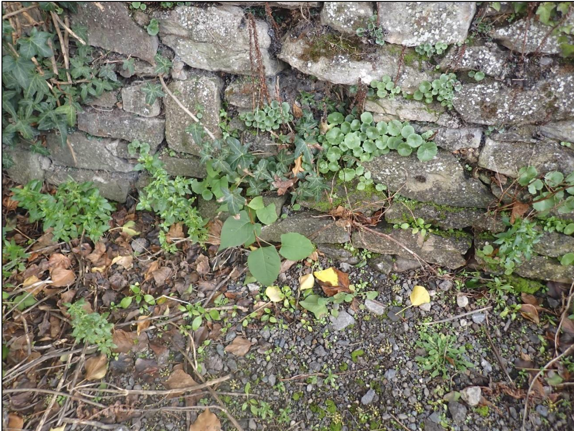
Plate 4-3: Single Japanese Knotweed plant growing from a stone wall to the south of the shed at the centre of the proposed development site.
