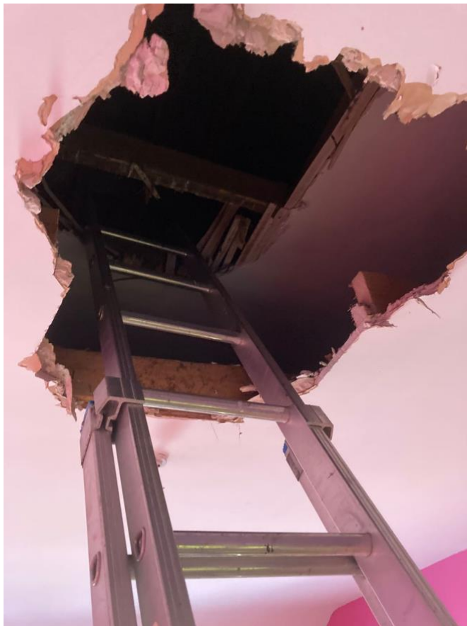
Fig. 1. Portion of ceiling removed by Leitrim County Council to allow access to attic areas
