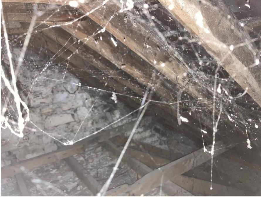
Fig. 3. Cobwebs on roof beams within attic.
