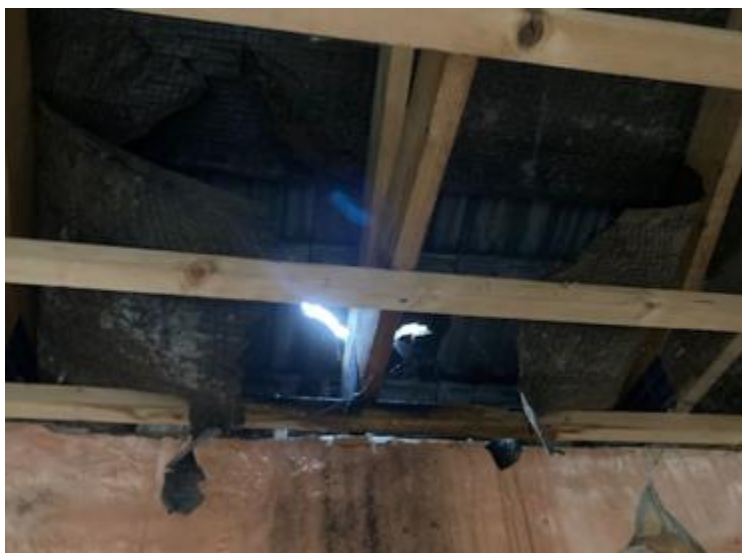
Figure 9. Gap in roof of function room.
