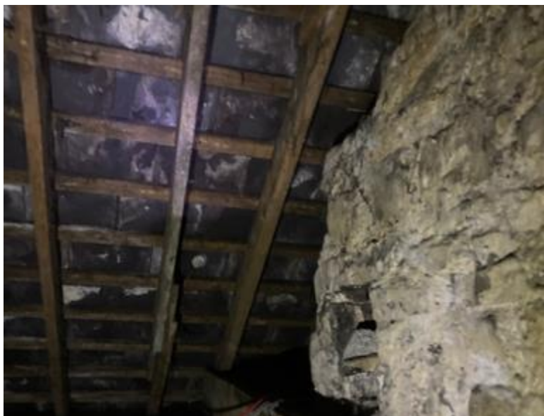
Figure 8. Attic space – the stone construction party wall shown to the right of photograph.
