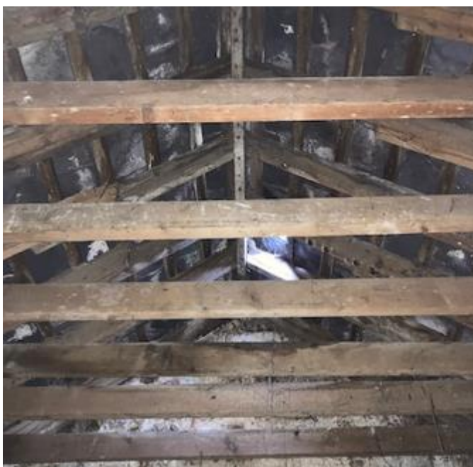
Figure 7. Attic space – note missing roof tile
