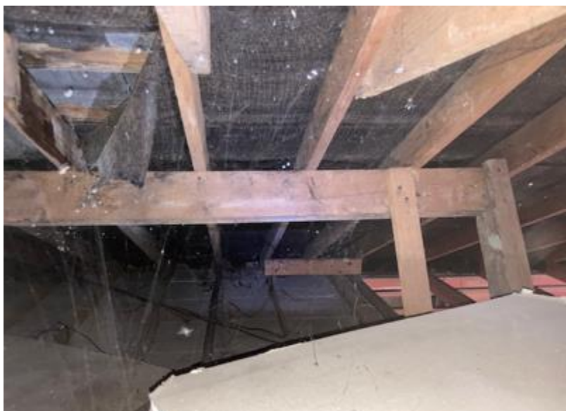
Figure 10. Roof space at rear of function room. Note abundance of cobwebs.
