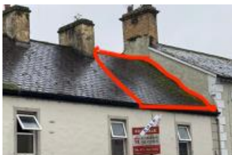
Figure 11. Section of roof where it is recommended that tiles be removed by hand.
