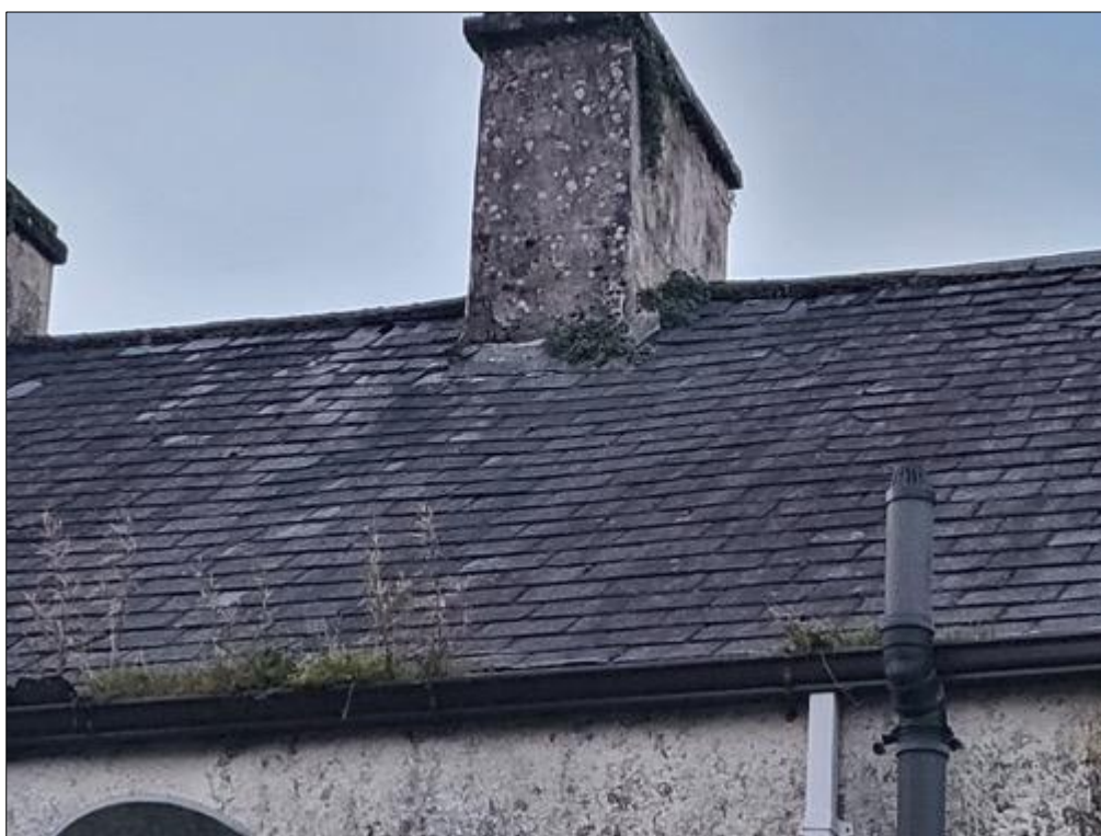
Figure 3. View of the building's roof, taken from the rear of the property.
