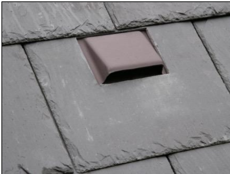
Figure 12. Example of an adapted roof slate that permits bat access to a roof space.
