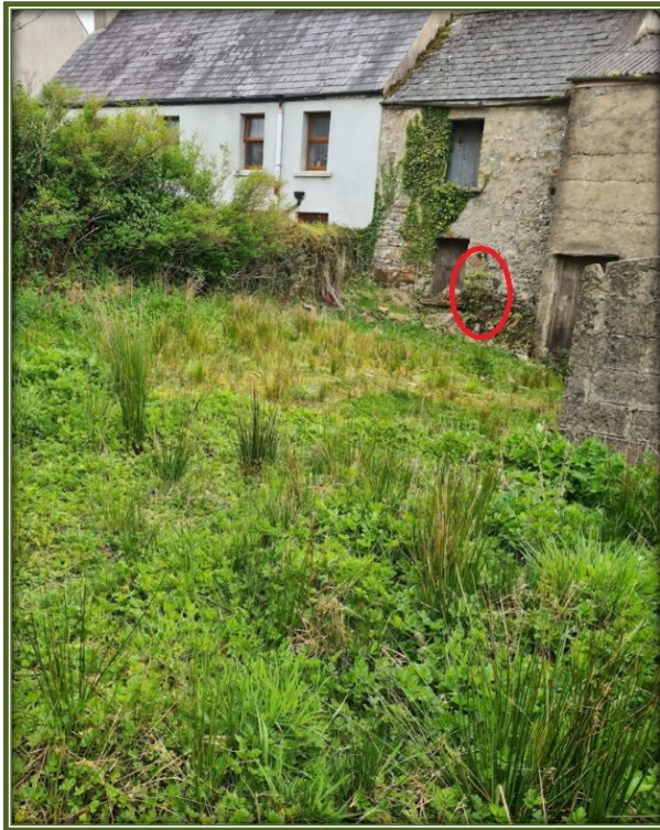
Photograph Showing Rear of Derelict Building and Location of Knotweed
