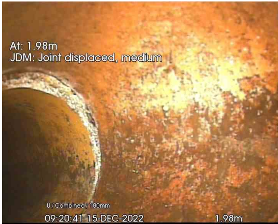
MH1 TO UPS2_1-98m_092041.jpg, 00:00:23, 1.98 m Joint displaced, medium
