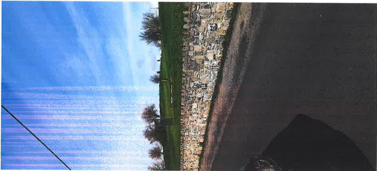
Traditional stone wall constructed on the western boundary to the Bohercrowe Road
